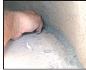
3. Place insulating-fibre blanket on foundation. Mortar inner edges of base with Refrax Mortar & position on blanket. Tap with rubber mallet to ensure good bond.
